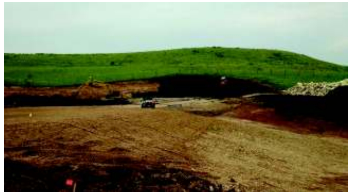
Applying 6"-8" of top soil on the slope behind the stone retaining wall of the parking lot, June 13, 2018.
