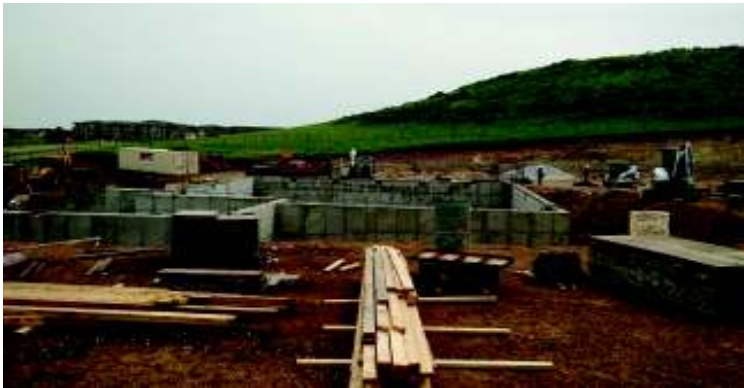
Poured concrete walls of lower level and east entrance to the lower level of the church, June 13, 2018. Standing at location of sanctuary.
